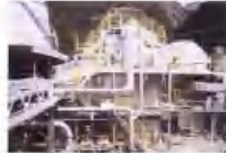
Wood Chip Burning Boiler
